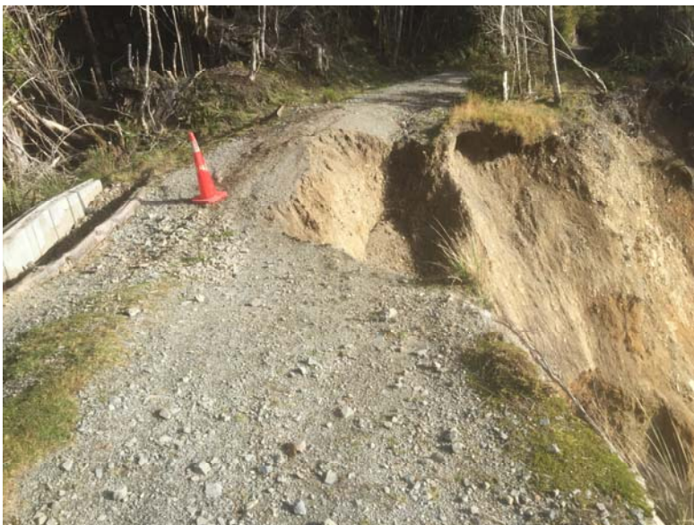
Chilly Creek Washout
